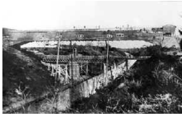
Original 247-foot span at Summit, Del., is dismantled, with new, lower replacement alongside. Note towpath at water's edge.
